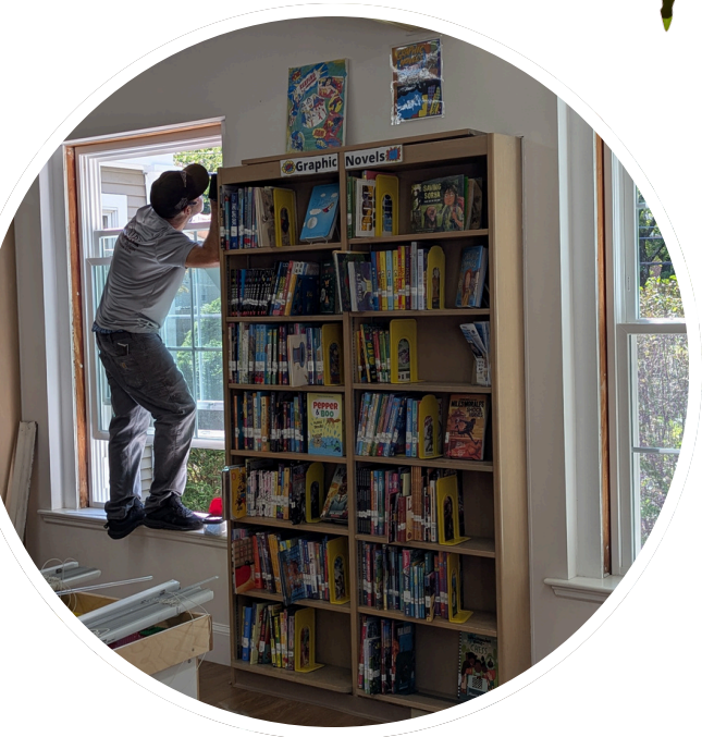
Venture Windows installed new windows in the children's room. The windows they replaced were from the original 1956 building. This project was paid for using funds raised at the Symphony of Sweets fundraiser.
